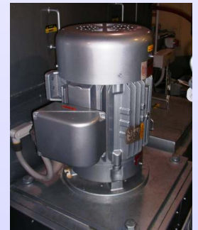
30 HP MAIN WASH PUMP
